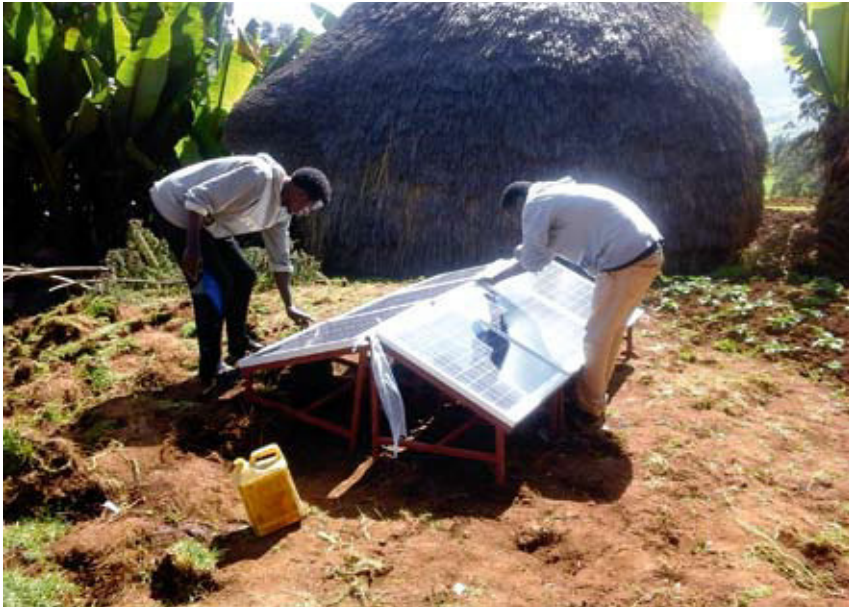
Solar installation in Laka
